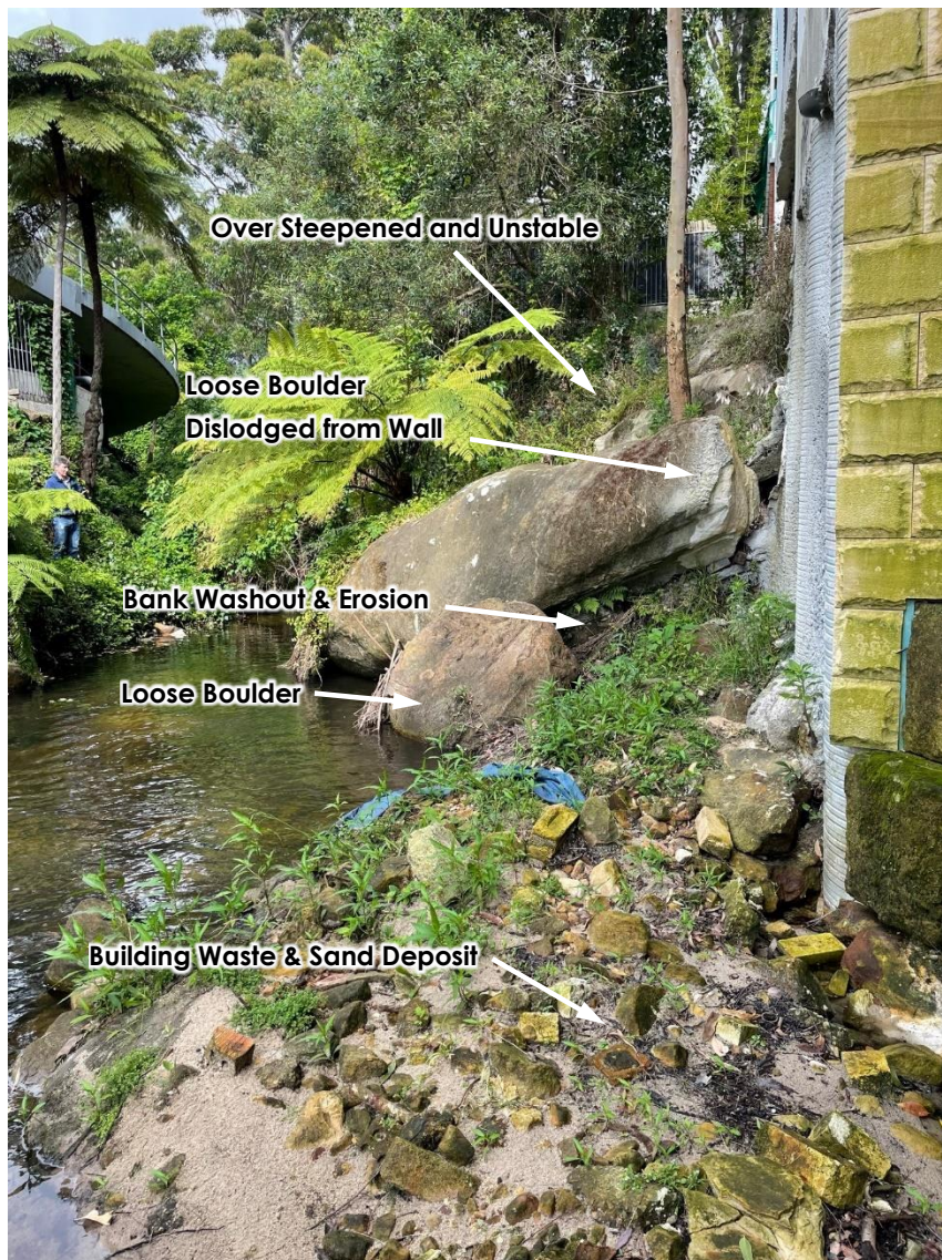
Figure 10: Northern Creek bank and embankment showing bank failure (17 November 2021).
